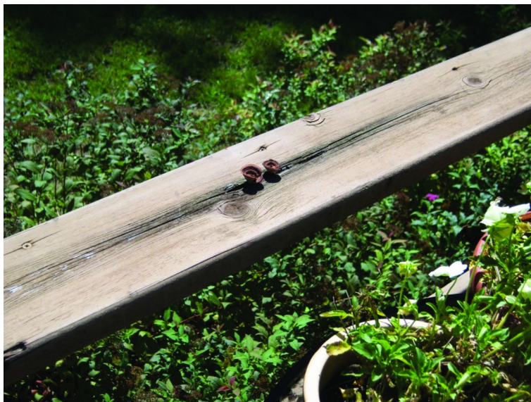
Figure 9. An example of how abiotic and biotic issues can work interactively to promote wood deterioration and destroy wood products in above ground outdoor exposures. Note the presence of an un-identified fruiting body protruding from crack in the board. (Courtesy of J. Winandy with permission.)
