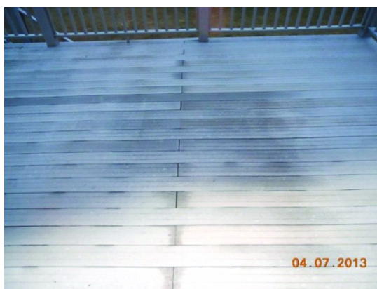
Figure 7. Wood-plastic composite deck boards after a rain shower followed by cloudy conditions. Moisture is retained for days within the decking, especially near joints where end-grain is exposed. (Courtesy of J. Winandy with permission.)
